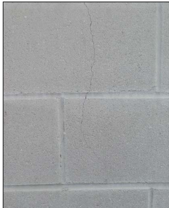
Fig. 5 Example Vertical Crack in South Wall of Target Store
