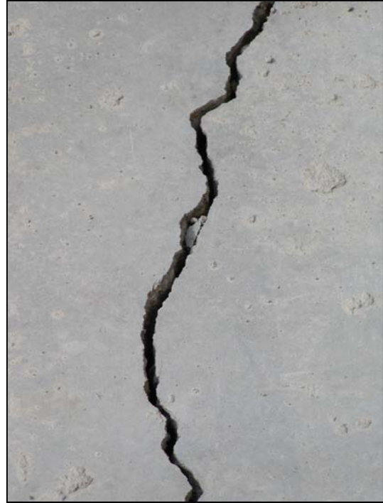
Fig. 4 Close-up View of Example Floor Slab Crack
