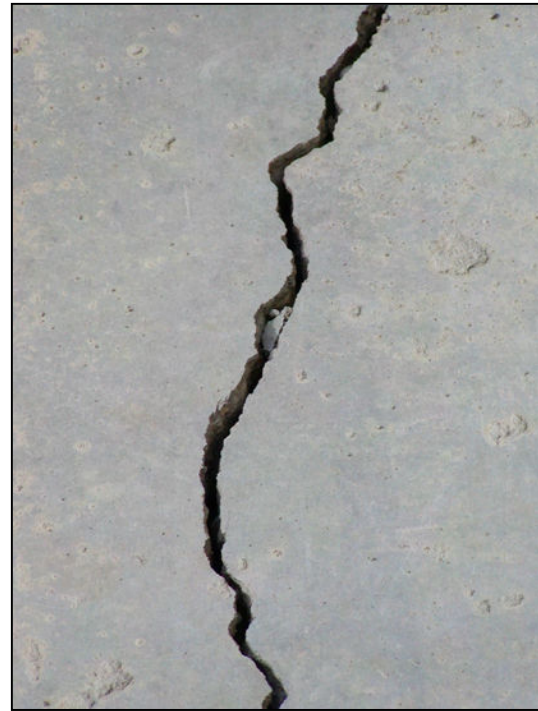
Fig. 4 Close-up View of Example Floor Slab Crack
